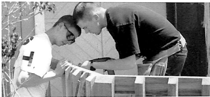
Jason Cory and Scott Mower work on a patio for a local resident as a class project.
